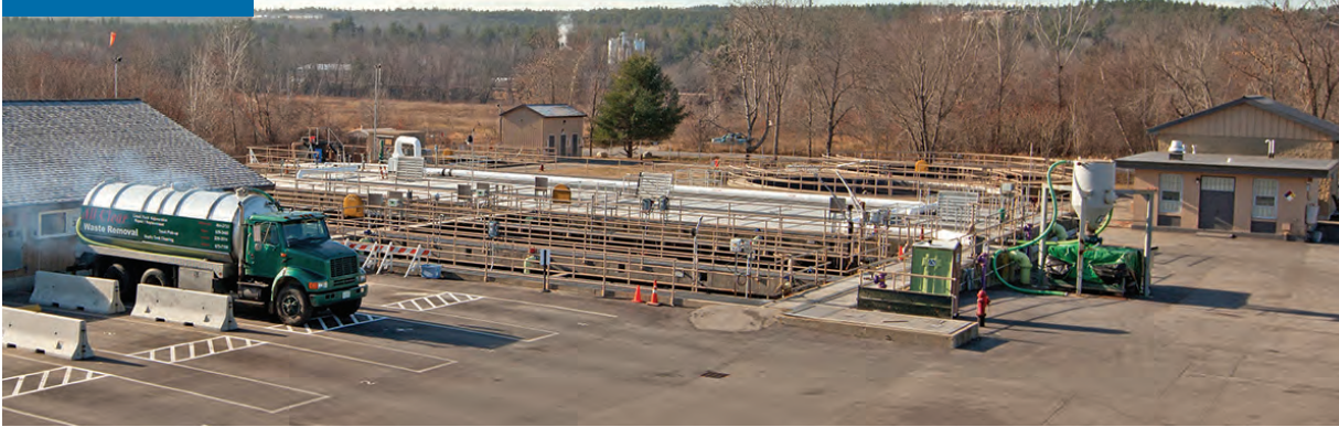
An overview of the Allenstown treatment plant. The small building on the right was the only plant addition needed to double capacity by way of the BioMag System.
